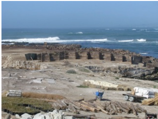
Figure 13. Photograph taken during construction of the Habitat Ridge and early plant restoration in 2010 (Carle et al., 2016)
